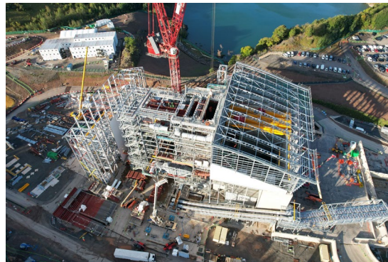
Newhurst EfW Facility
