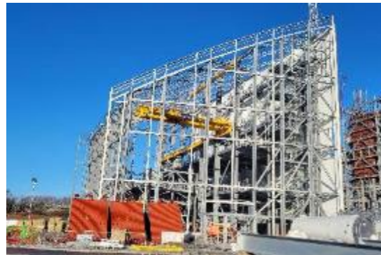
Skelton Grange EfW 2024 Industrial Award Winner, Tekla Awards 2025 Structural Steel Design Awards - Shortlist
